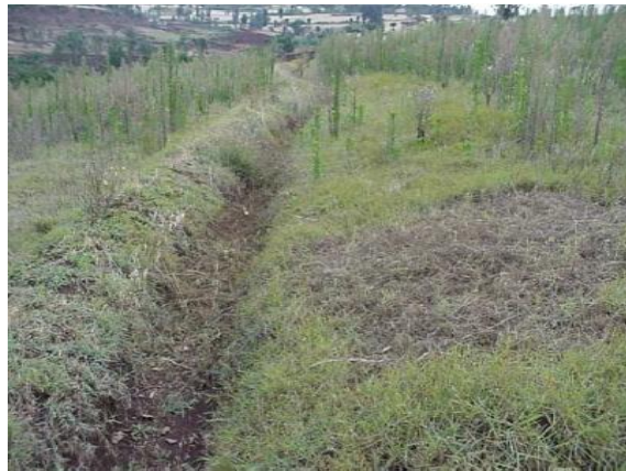
Photo 3: Cut-off drain placed on the upper part of cultivated land to protect soil bunds and farm lands from excess runoff
